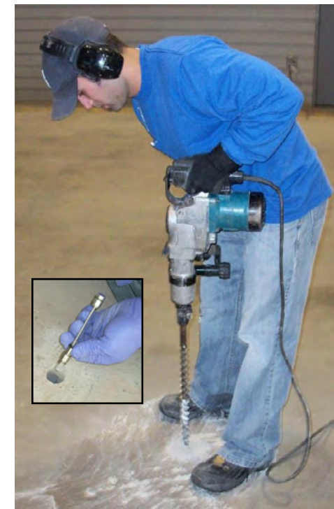
UNDER THE FOUNDATION: A vapor intrusion expert drills into a foundation slab before installing a vapor probe (inset). The probe was installed as part of vapor intrusion sampling efforts that occurred in January and February.
