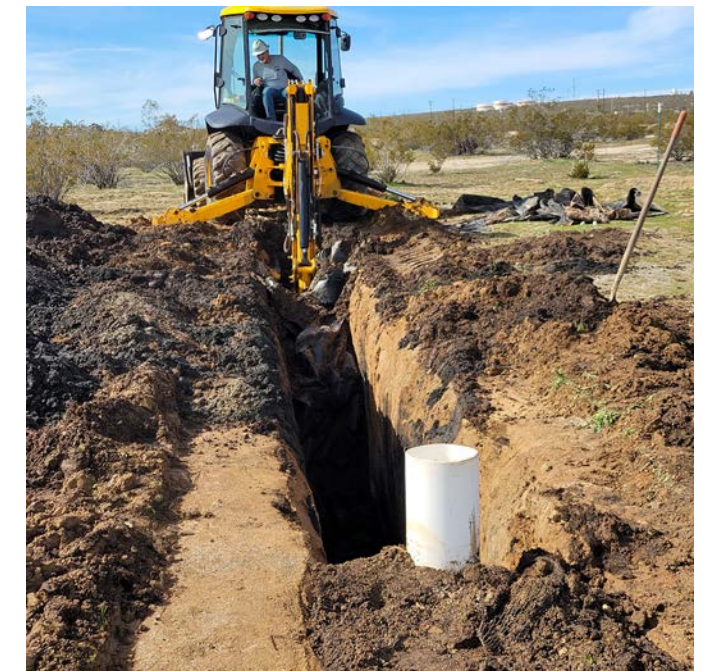
RESTORING THE SITE: In February 2024, excavation and final grading of all three trenches to restore the site to its initial state was completed.
