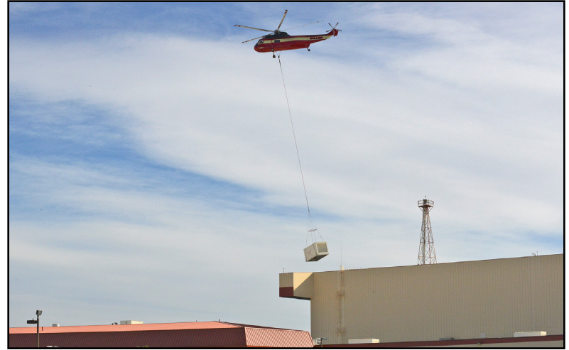
An S-61V Sikorsky helicopter lifts an old cooling unit off of Bldg. 1600 April 7 to be placed down at a parking lot nearby. (U.S. Air Force photo by Kenji Thuloweit)
